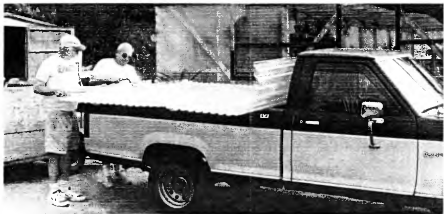
Carl McLeod, in a rare moment without his straw hat, working with and Stan Yalof on Baja Greenhouse roofing project in 1998.
